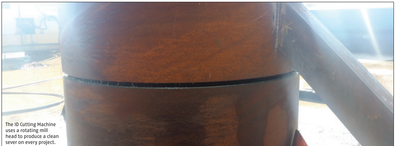
Installing the ID Cutting Machine by lowering it down to the inside of the pile to the cut line located at the mudline.
